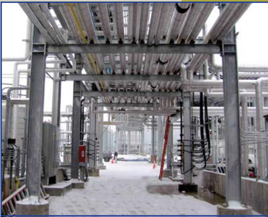
The Lake Erie Biofuel Plant is one of the top ten alternative energy production facilities in the nation.
