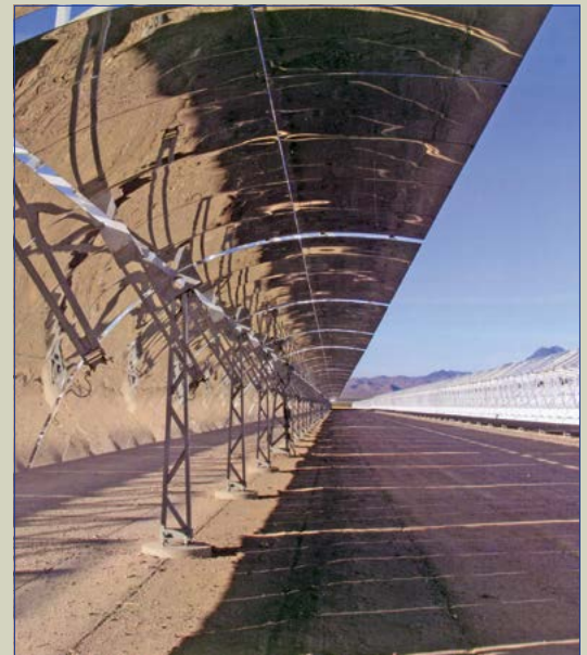
Sixty-four megawatts of power will be generated by the 180,000 mirror panels in the farm.
