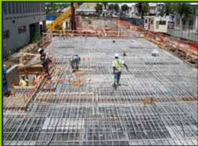
The Magistrate Court and Hamilton Police Station in Bermuda have their foundations set in galvanized steel rebar.
