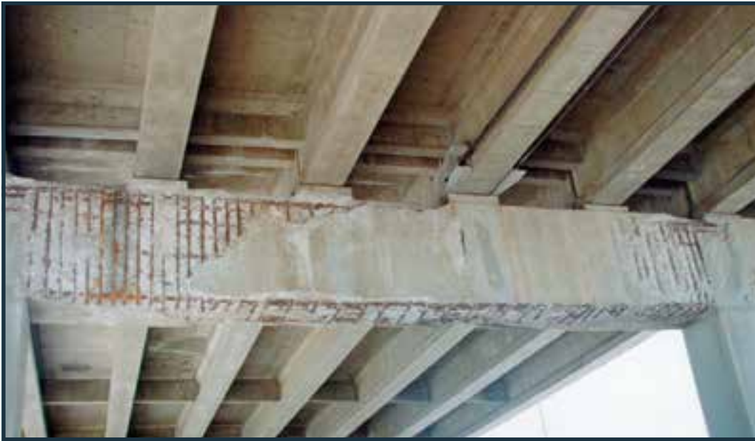
Corroded rebar causing concrete spalling
