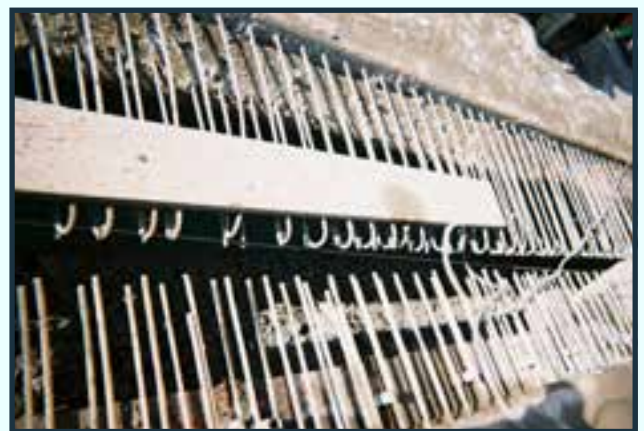
The galvanized rebar from the Route 66 Bridge Deck in Kittanning, Pennsylvania, after more than 30 years of service.
