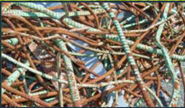
Rusted epoxy-coated rebar
