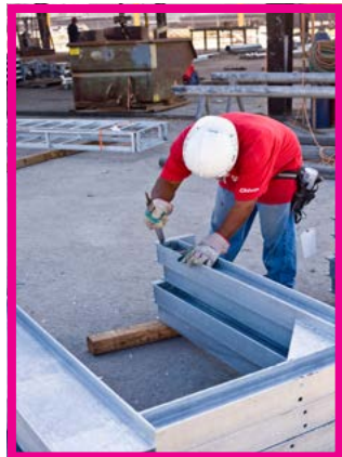
Workers prepare the galvanized surface for powder coating by filling any bumps, runs, or drips created during the galvanizing process.
