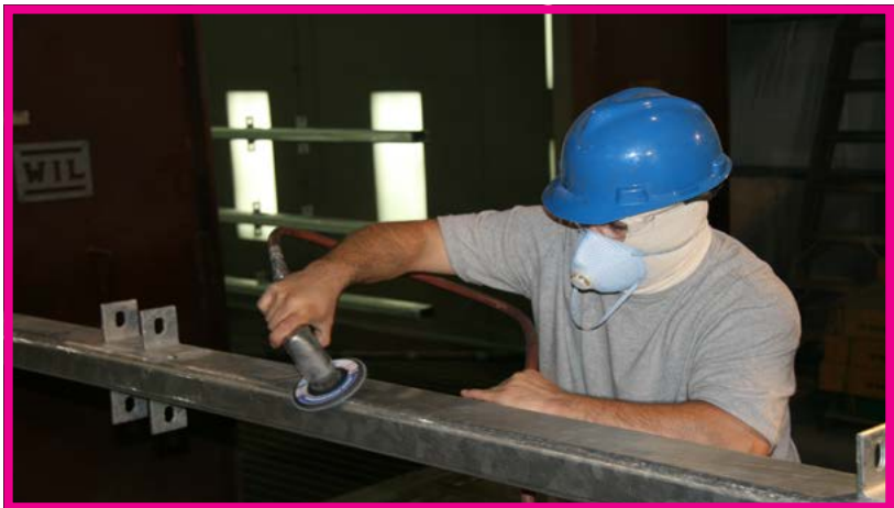
Grinding roughens the surface to make a good anchor for the powder application and adherence.
