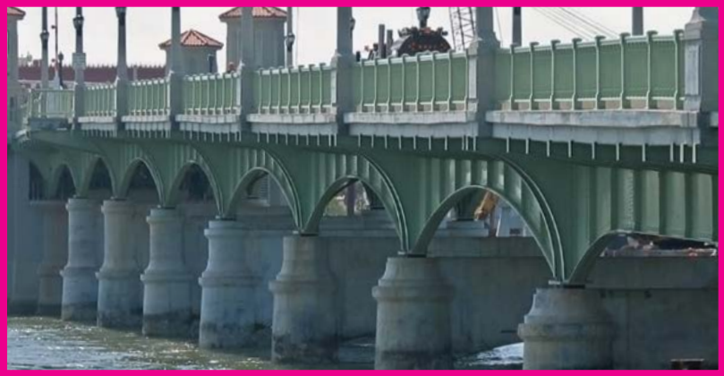
The Bridge of Lions in St. Augustine, Florida, utilizes a duplex system of powder coating over hot-dip galvanized (HDG) steel for corrosion protection.
