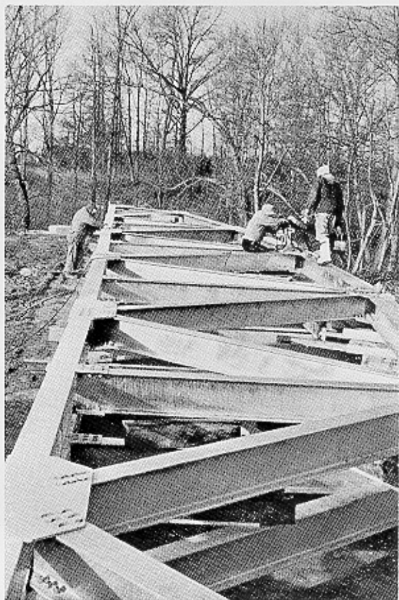
HOT-DIPPED GALVANIZING of the steel used on the Montgomery Road bridge offers both barrier and cathodic corrosion protection that county officials felt would not have been achievable by painting the steel structure.
