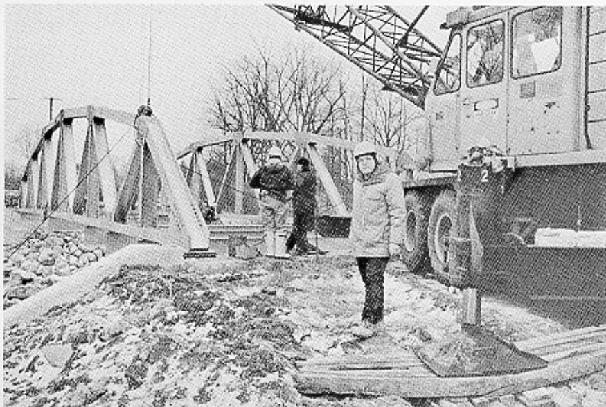
WORKERS ARE SCHEDULED to build three more galvanized steel bridges like the Montgomery Road bridge in Ashtabula County, Ohio, by the end of 1991.
