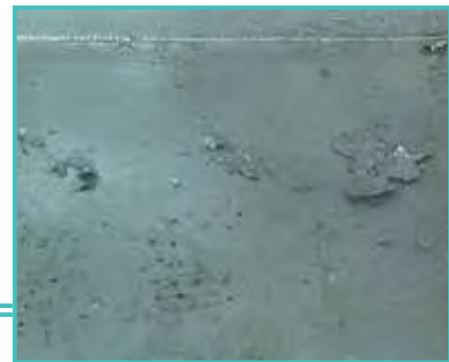
FIGURE 38: ZINC SPLATTER (ACCEPTABLE)
