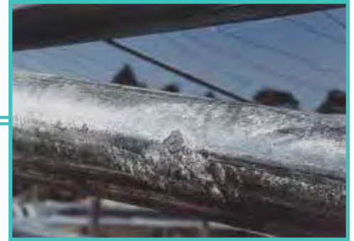
FIGURE 25: TOUCH MARKS (REJECTABLE)
