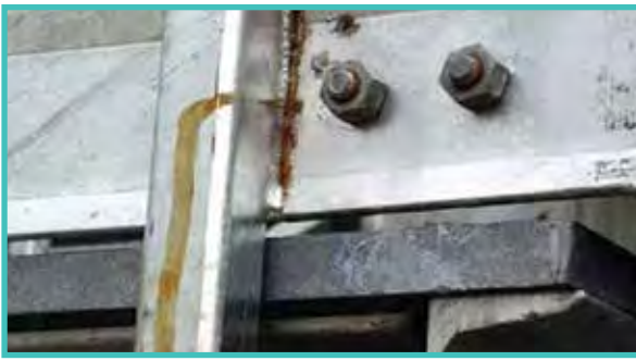
FIGURE 28: RUST BLEEDING (ACCEPTABLE)
