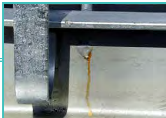
FIGURE 33: WEEPING WELD (ACCEPTABLE)
