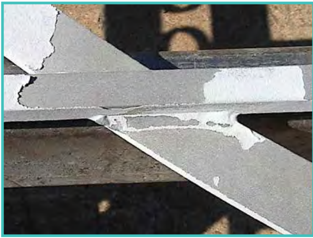
FIGURE 13: BLASTING DAMAGE (REJECTABLE)
