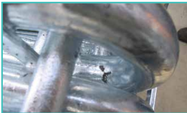
FIGURE 12: BARE SPOTS (REJECTABLE)
