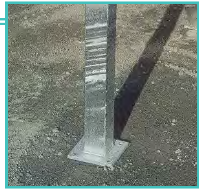
FIGURE 23: OXIDE LINES (ACCEPTABLE)
