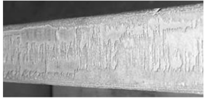
FIGURE 12: EXAMPLE OF HDG COATING APPEARANCE FORMED OVER UNPREPARED FLAME-CUT EDGE
