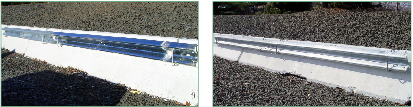
FIGURE 14: NATURAL WEATHERING OF WET STORAGE STAIN
