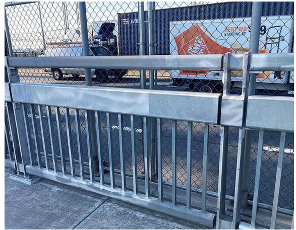
WEATHERING OF REPAIRED MATERIALS
