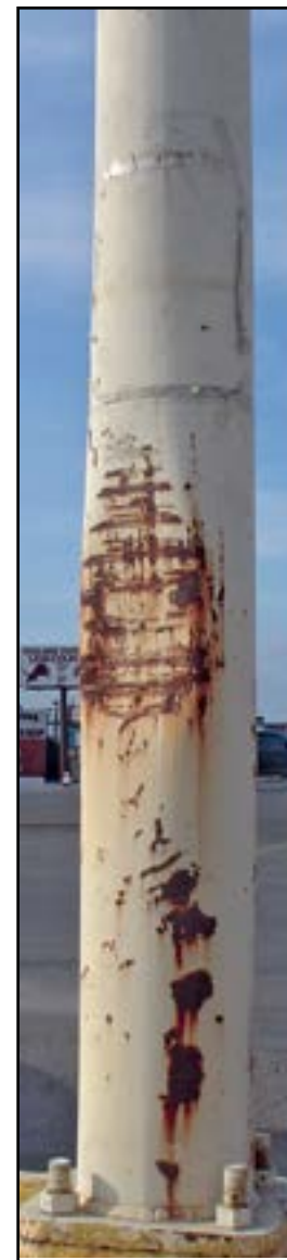
Corroding painted pole
