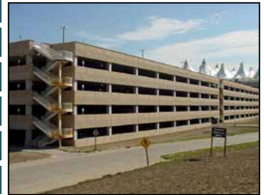
Painted Parking Garage Stairs after (8 years of service)
