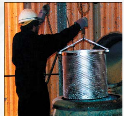
Fasteners in perforated basket are removed after being spun to remove excess zinc.
