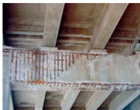
Figure 1 Spalling concrete under bridges signifies a deteriorating structure and presents a safety hazard for traffic below.
