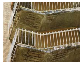
Figure 2 Black reinforcing bars are exposed by spalling concrete on the underside of these stairs. This unsightly deterioration is unsafe for people to use.
