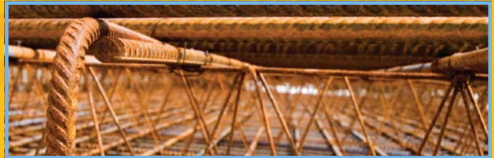
Corrosion is not only unattractive, but structurally damaging and dangerous, as well.
