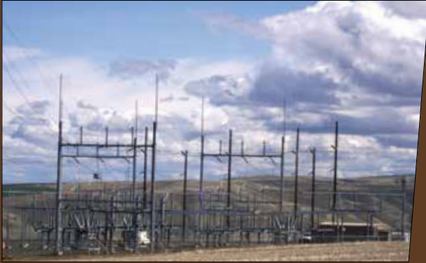
Talbot Substation Dayton, Washington
