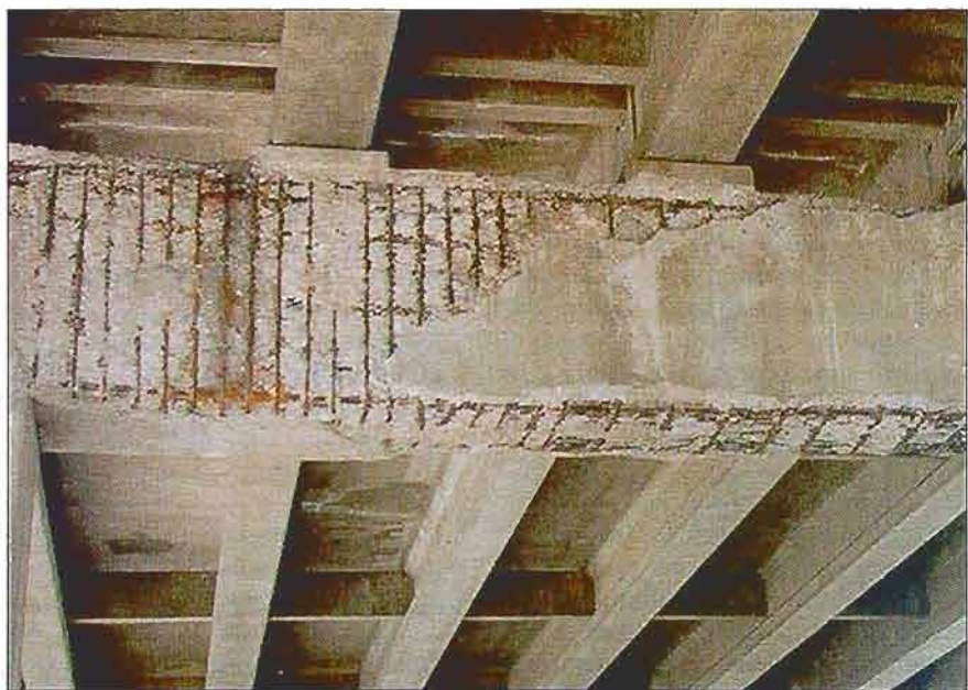
The development of dense corrosion products on the surface of black (uncoated) rebar builds up pressure against the surrounding concrete. When these expansive forces elevate to a level that exceeds the strength of the concrete, cracking and spalling occur, ultimately resulting in failure.
