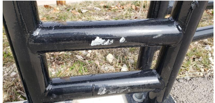
Figure 4: Paint Removed from Center of Rail
