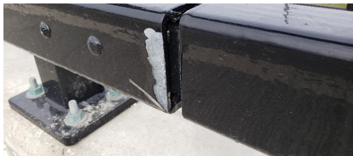
Figure 2: Paint Removed from Bottom of Rail
