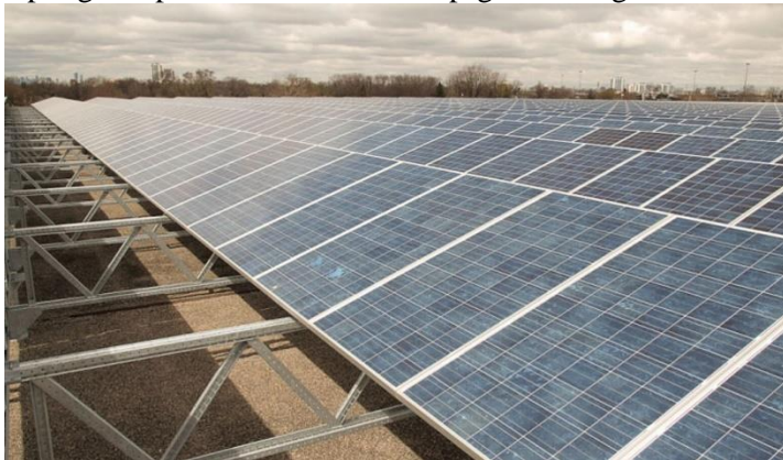
Fig. 5. Metropolitan Tea- 702 kW Solar PV Installation-Toronto, ON
